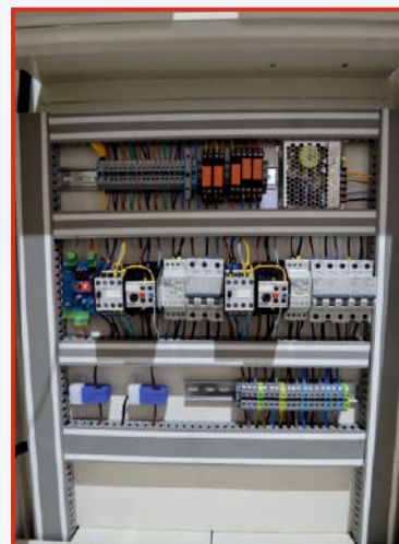
Internal part of the control panel
